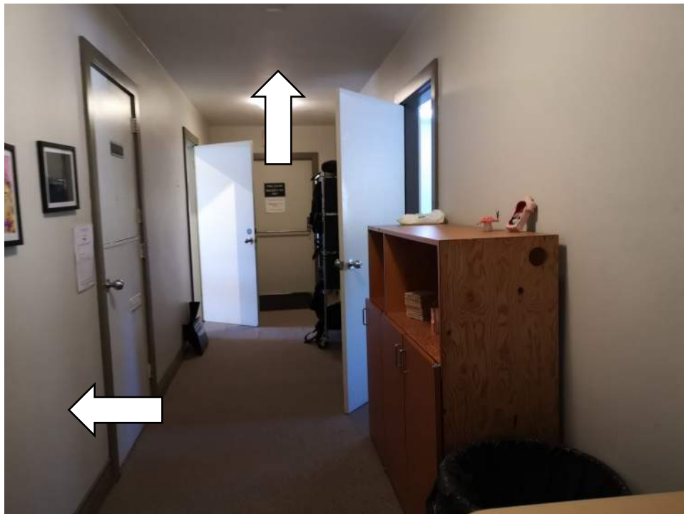
Photo - C30 00 00.01 - Interior Finishes - Wall and Ceiling Repainting / Hallways, Offices and Classrooms
