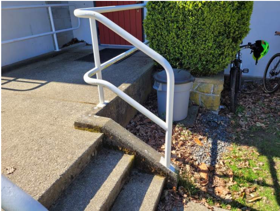
Photo - G20 30 03.02 - Hard Landscaping - Concrete / Walkways and Patios / At The Rear of the Building
