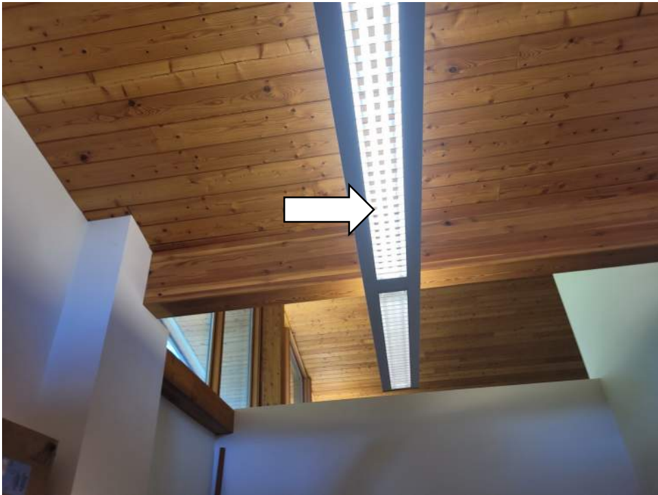
Photo - D40 20 02.02 - Interior Lighting - Replacement / Narthex
