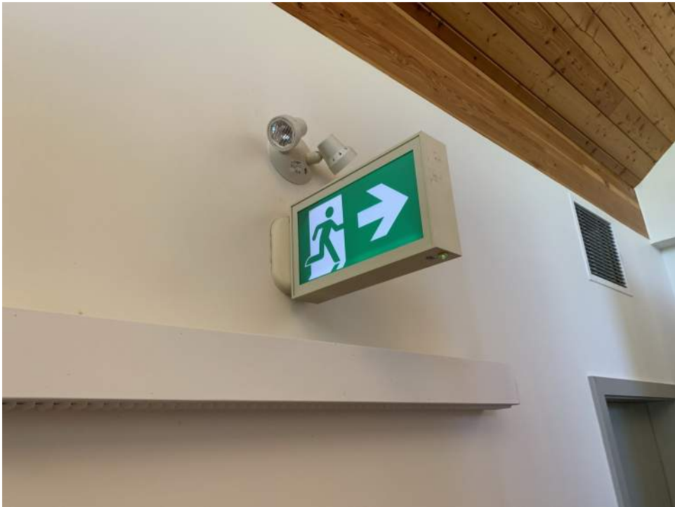
Photo - D40 20 08.00 - Emergency and Exit Lighting - Replacement / Paths of Egress
