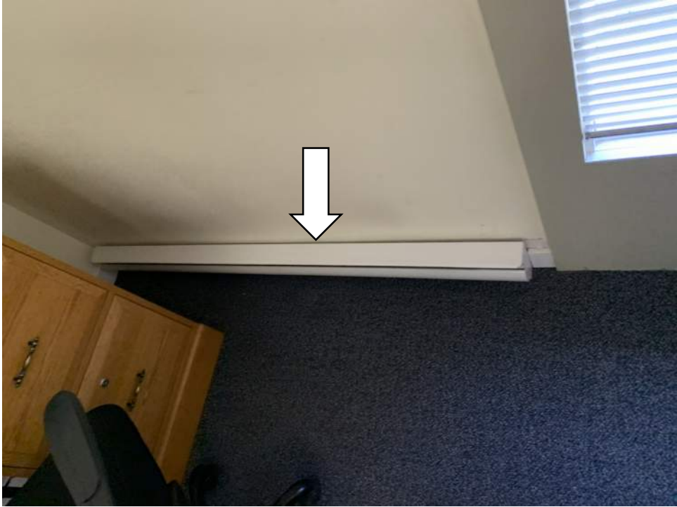
Photo - D30 50 06.01 - Electric Baseboard Heaters - Replacement / Office, Classrooms, and Lower Hall Area
