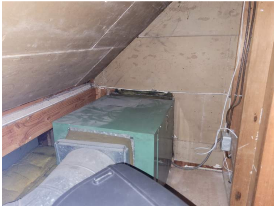
Photo - D30 40 08.00 - Air Handling Unit - Replacement / Upper Floor Office, Storage Space - Under Sloped Roof
