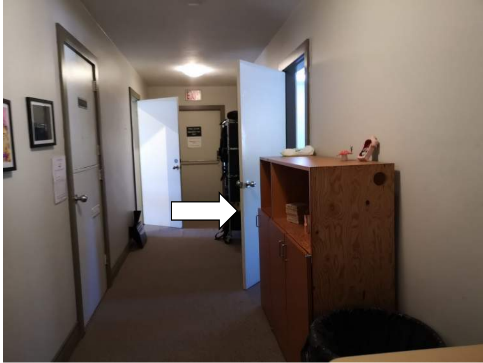
Photo - C10 20 03.00 - Interior Doors - Repairs / Office, Classroom, Utility Spaces and Common Areas
