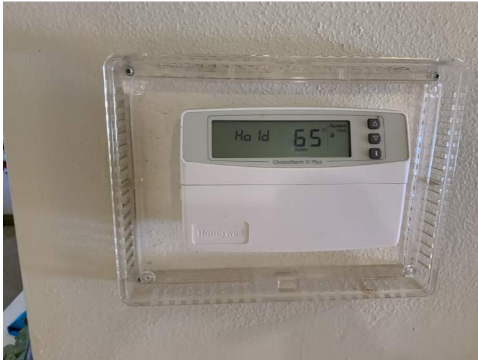
Photo - D30 60 02.00 - HVAC Controls - Replacement / Throughout
