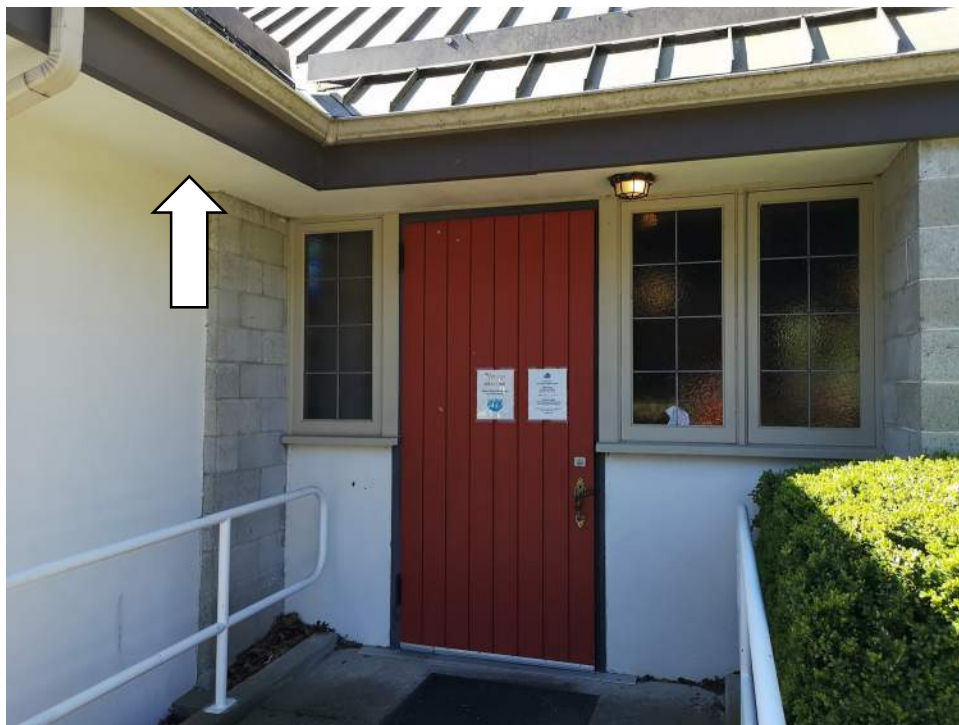
Photo - B20 10 08.01 - Soffits - Repaint and Repair / Roof Overhangs / Original Church
