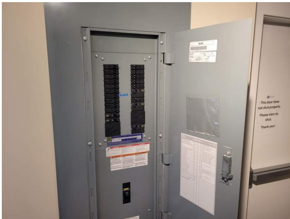
Photo - D50 10 05.00 - Branch Circuit Panels - Replacement / Office Area and Men's Washroom
