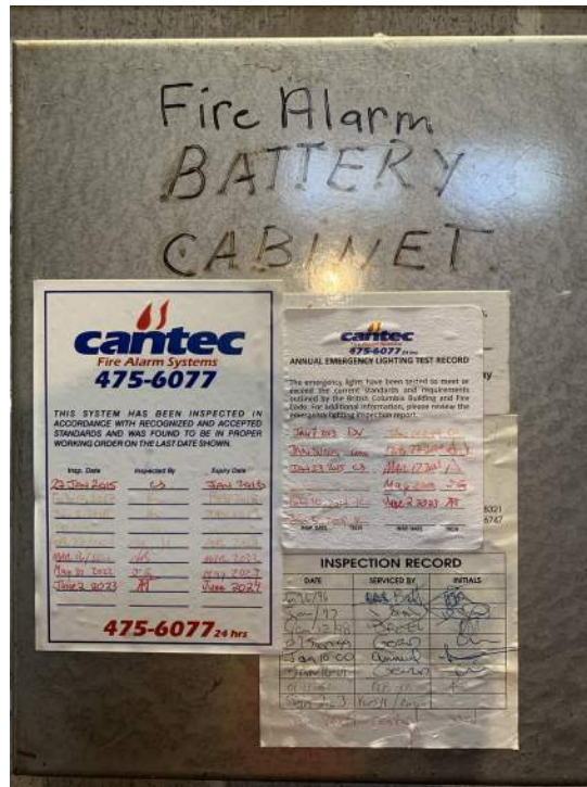
Photo - D50 30 01.00 - Fire Alarm System - Replacement / Throughout
