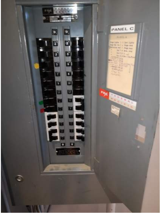
Photo - D50 10 05.00 - Branch Circuit Panels - Replacement / Various Locations
